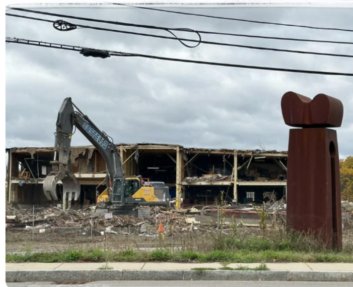
Nashua Priority Project Nimco – Demolition of the former Nimco site in Nashua began in 2025. This former brownfield site will be redeveloped into housing. Photo credit to city of Nashua.
